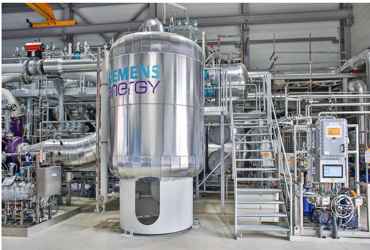
Figure 5: Large river-water heat pump in Mannheim, Germany (Source: GKM, Case study details in: IEA TNCG, 2025)
