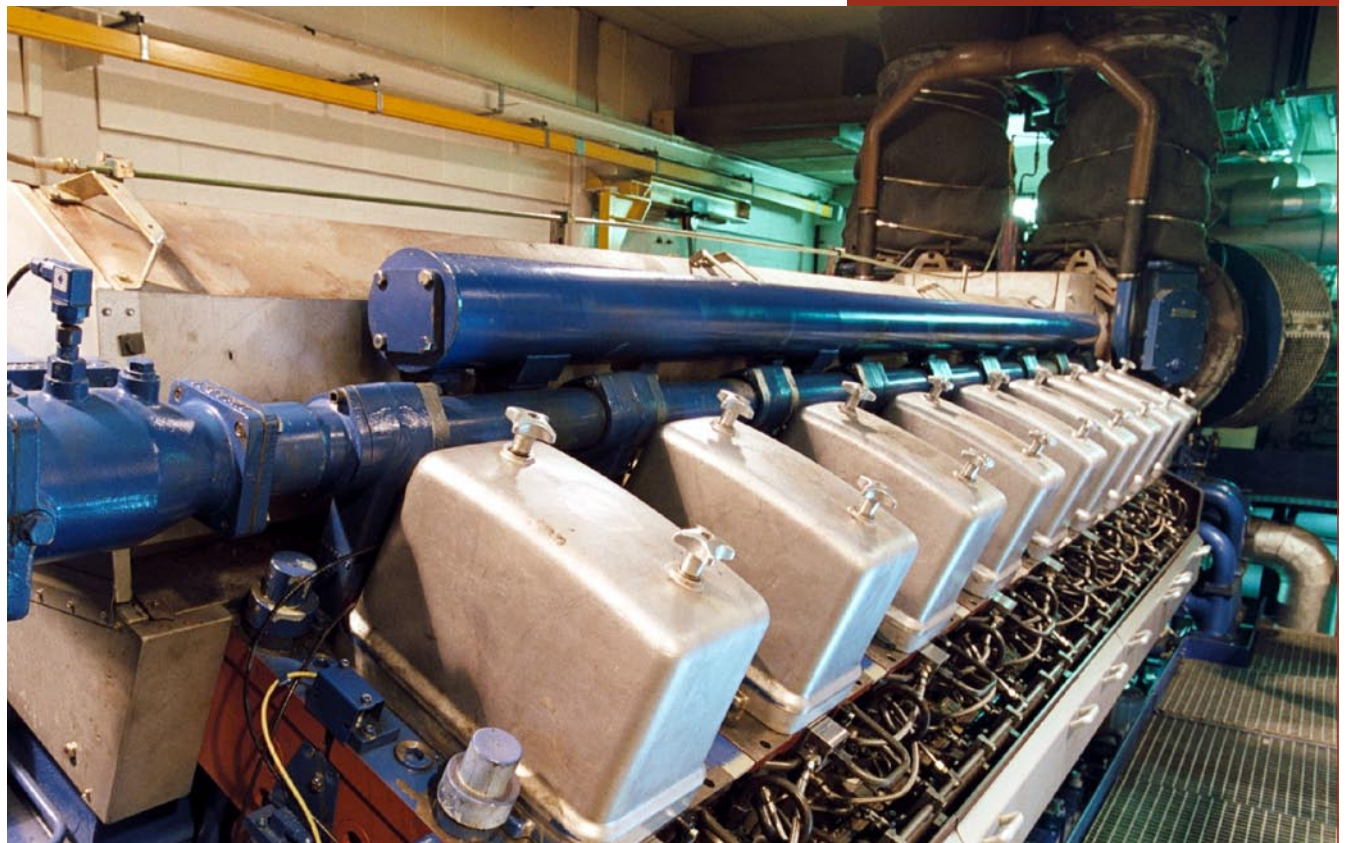
Southampton's 5.7MW e CHP Engine (below)
