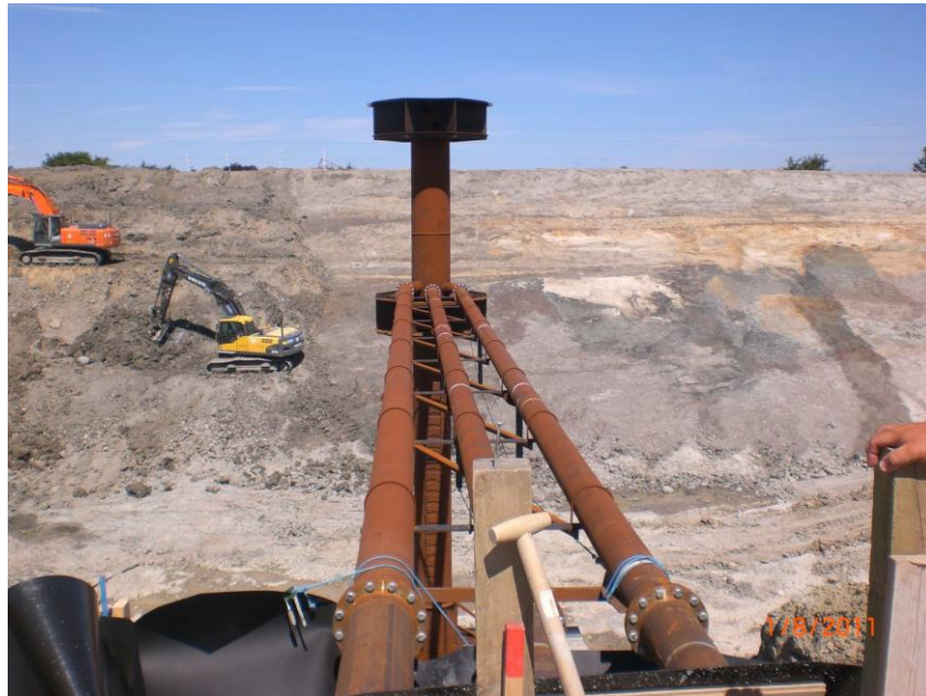
Figure 4.14: In-/outlet arrangement led through the side of the storage. Photo from the implementation of the SUNSTORE 4 storage in Marstal (Marstal Fjernvarme)
