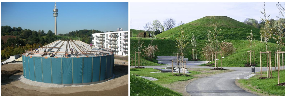
Figure 2.3: Tank thermal energy storage with 5,700 m 3 of water volume built from prefabricated concrete elements in Munich, Germany (in construction and finalized, Solites)
