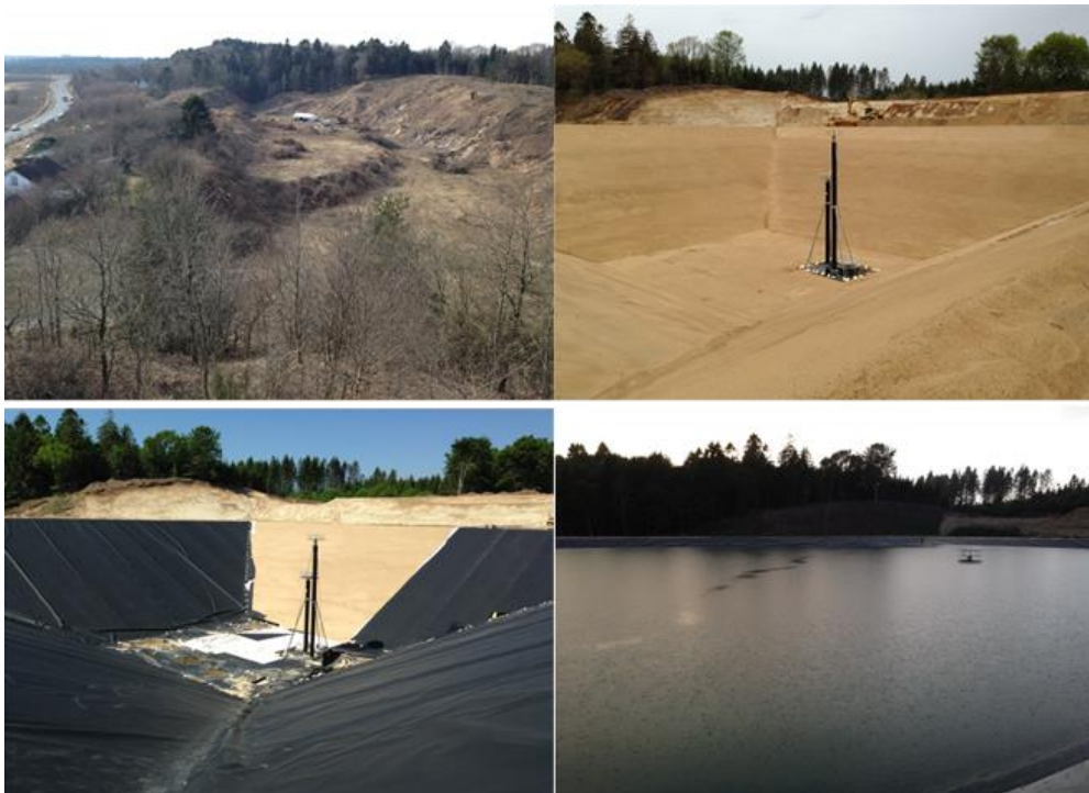
Figure 5.10: Pictures from implementation of the pit heat storage in Dronninglund (source Dronninglund Fjernvarme)
