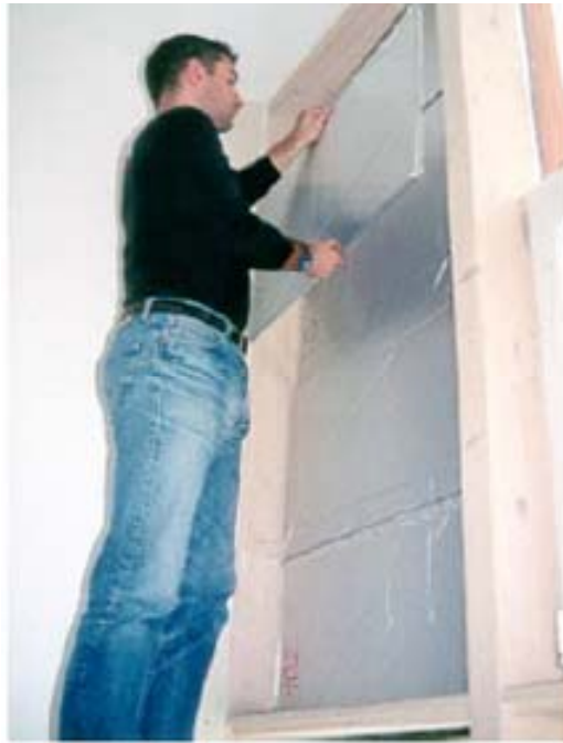
Figure 26: Installation of vacuum panels in the southern facade of the new ZAE building.
