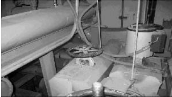
Figure 4.1-13: Bypass valve as part of the installation in C17 (large valve with steering wheel)
