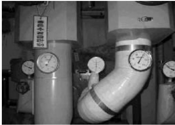
Figure 4.1-12: The temperature status of DHW (the secondary DHW supply temperature is 90°C)
