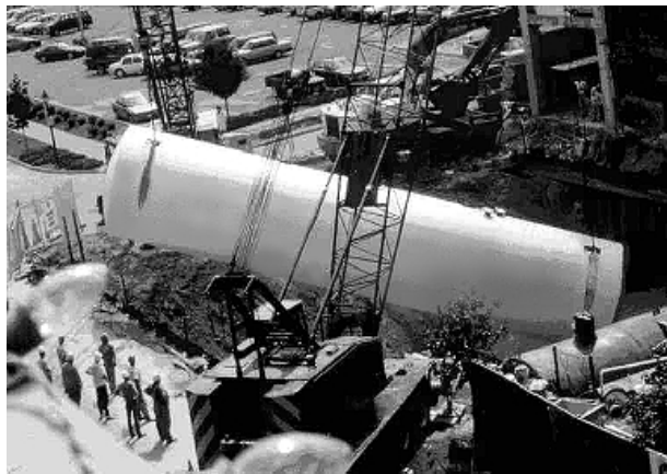
Figure 25 Pressurized storage tank for a hospital. (Source: Cryogel)
