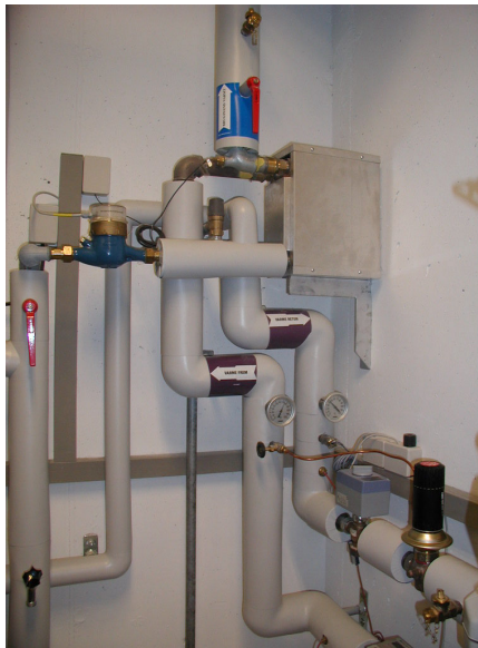
Part II Figure 11.1: Heat exchanger for hot water supply in an office building connected directly to the DH system
