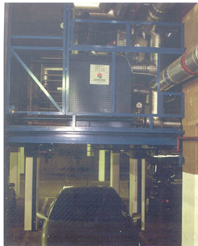
Part II Figure 10.10: Heat exchanger substation located above a car park bay
