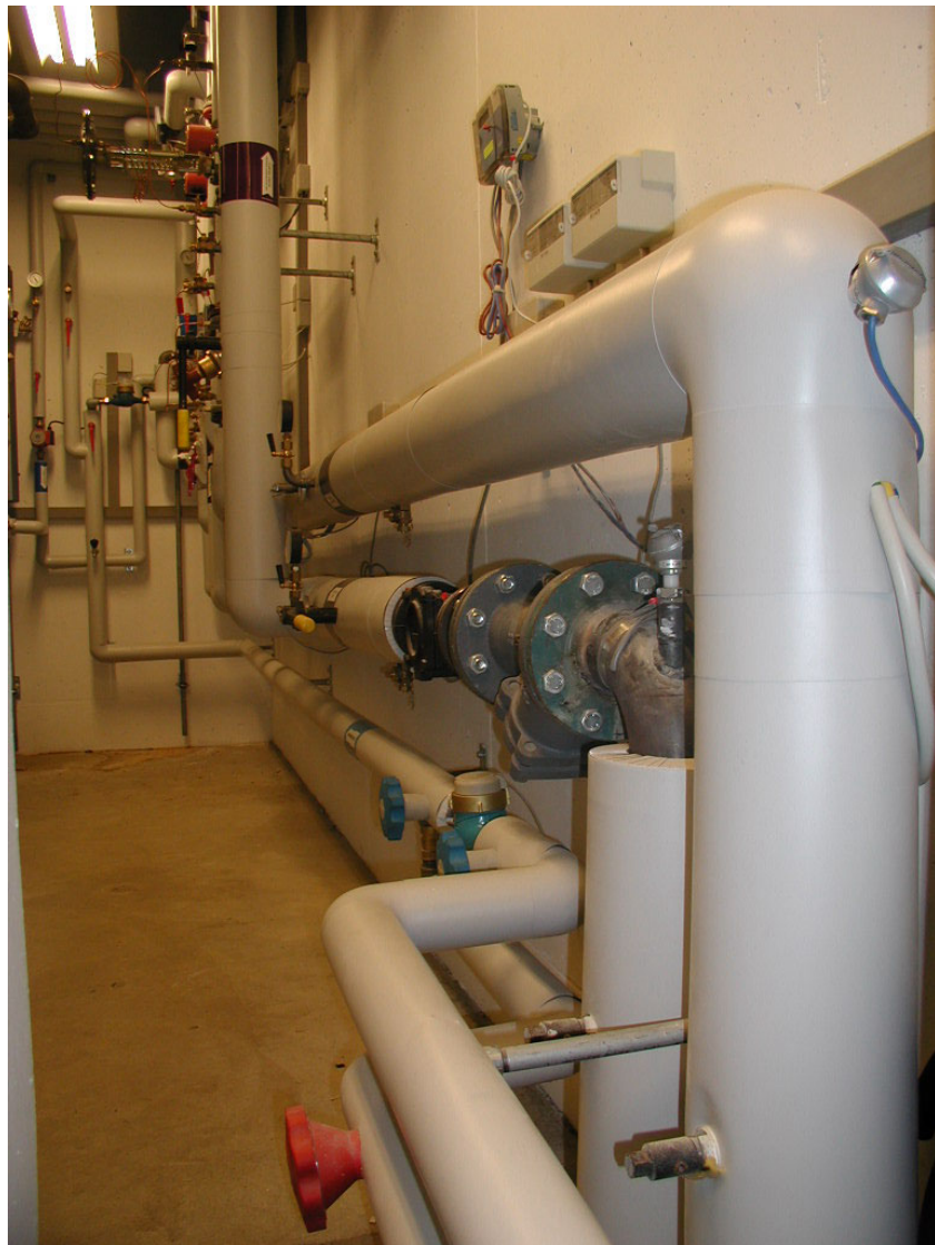
Part II Figure 10.9: Directly connected installation. The main pipes are coming into the building in the foreground
