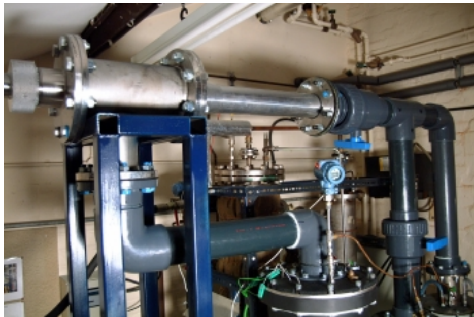
Figure 5: A close-up view of test rig showing jet-pump connected to plastic suction and discharge pipes fitted with 4 inch nominal diameter (101.6 mm) plastic ball-valves.
