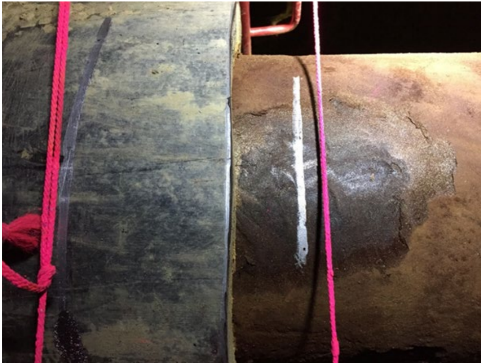
Measurement of the relative movement between the steel pipe and the PE casing for the purpose of proving the defective bond 2013/14, source: EVN
