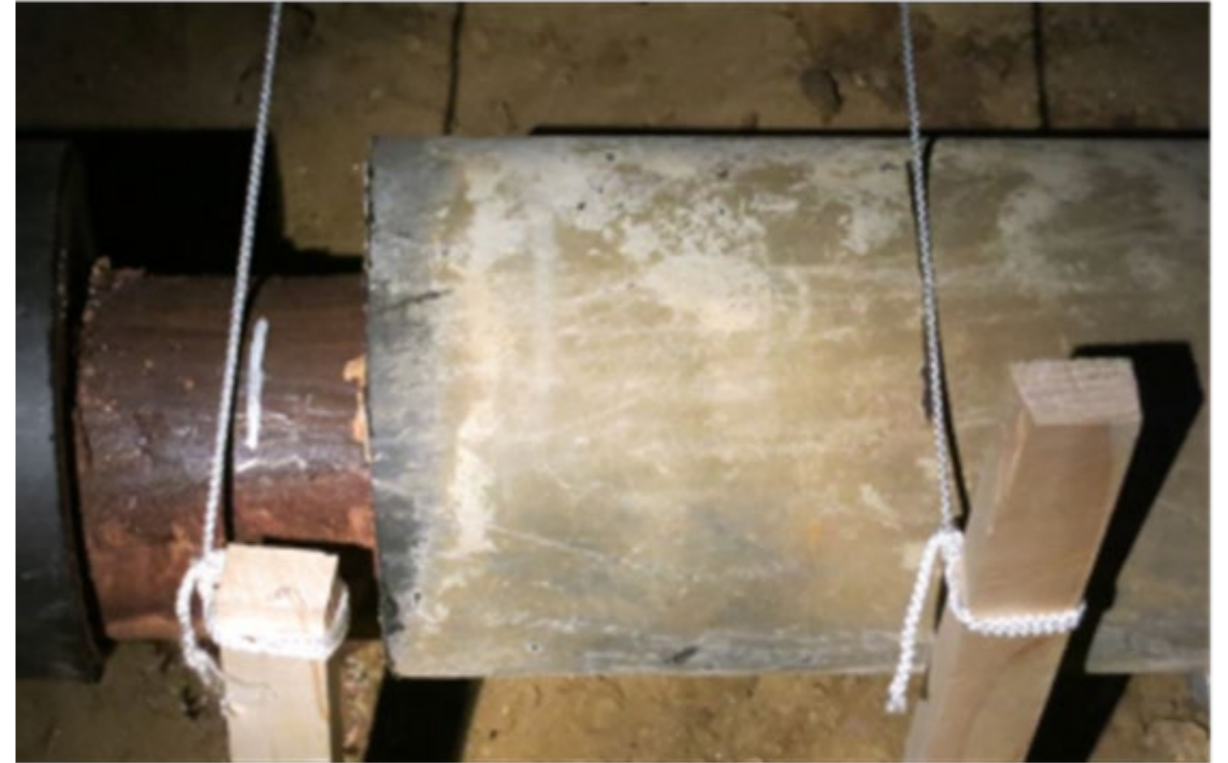
Measurement of the relative movement between the steel pipe and the PE casing for the purpose of proving the defective bond 2013/14, source: EVN
