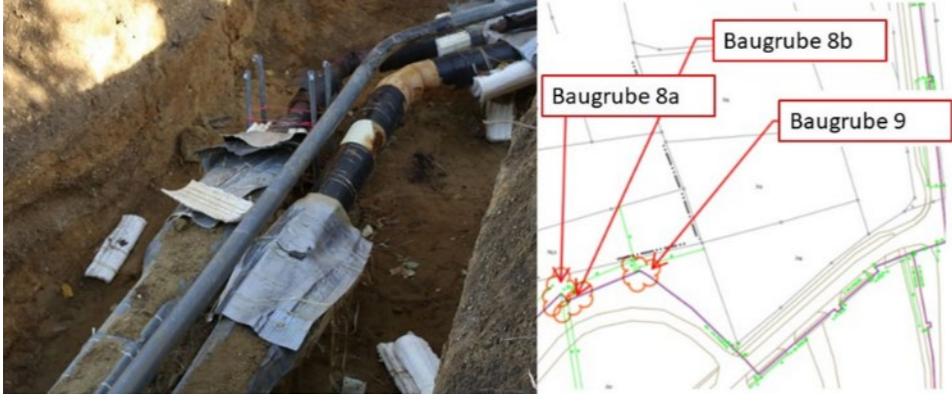
Left: Extraction Point 9, right: Sketch of the extraction points in DH network
