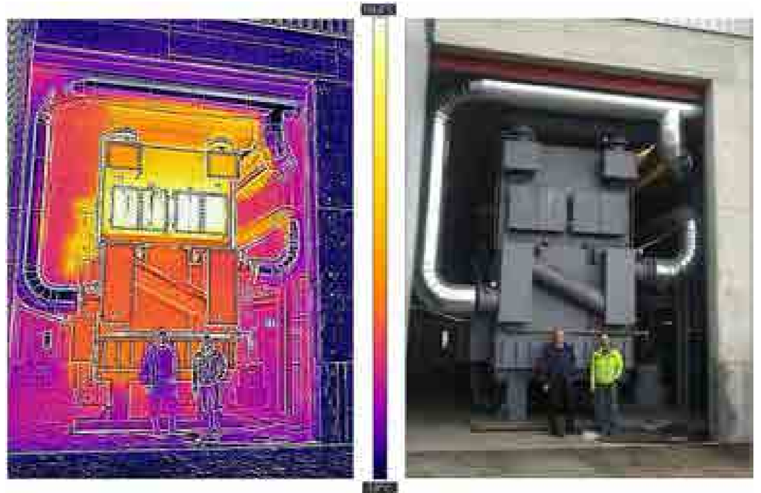
23 MW Absorption Heat Pump, Austria, 2018
