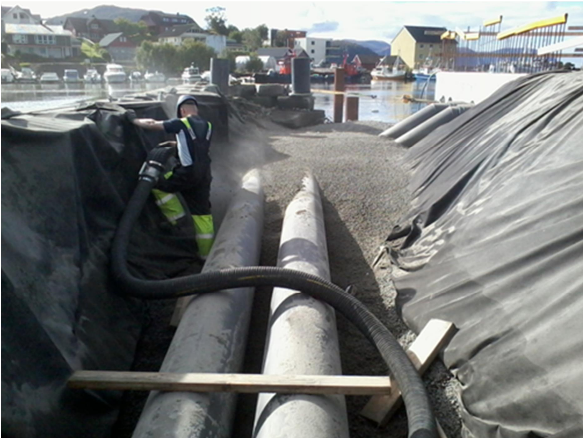
Figure 31. Pipelines for supplying water used as a heat source for heat pumps in a district heating system in Ulstein. (Photo, Øyvind Amdam, Ulstein municipality)
