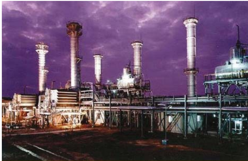
CHP Plant: Arvind Textile Mill, India
