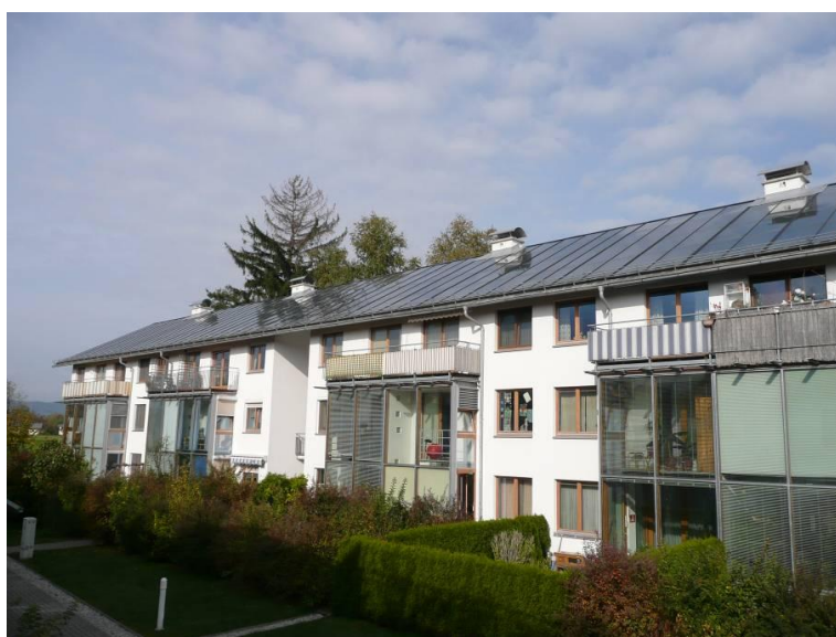
Figure 123. Solar collectors, pellet furnace and air conditioning with heat recovery in a low energy building. Salzburg, Austria. (Photo Benny Bøhm)
