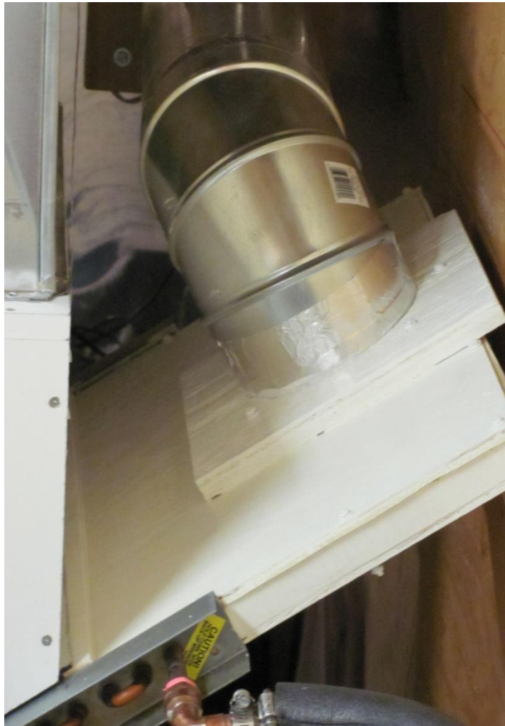
Figure 13: View of Extended Plenum from the Top Coil
