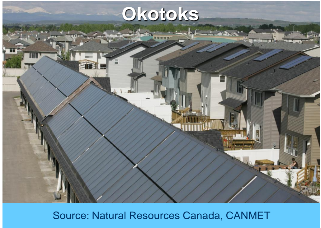
Figure 2: Solar Collectors on Garage Roofs in Okotoks
