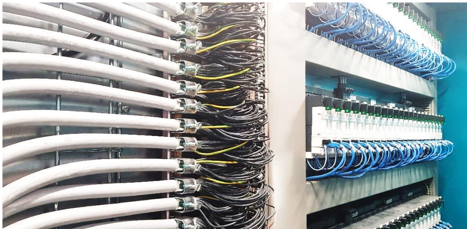
Figure 5. Small section of the electric hardware for a large-scale heat pump. Though the installation can be complex, the revenue from enabling optimized (possibly remote) operation may be substantial.
